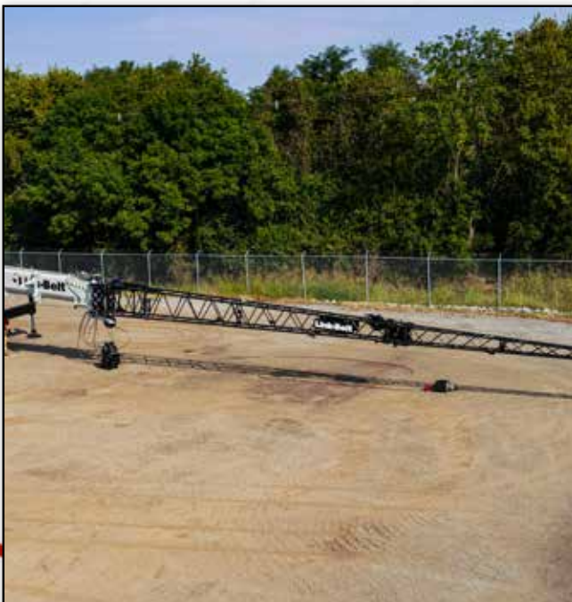
New fly erection & ground control system minimizes work at height.
